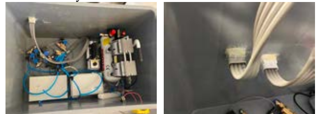
Figure 5. Pipes and Connectors
